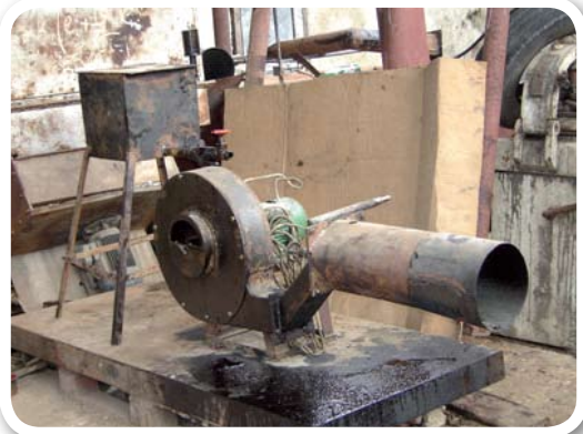
Photo showing HFO Burner with Fuel Tank
